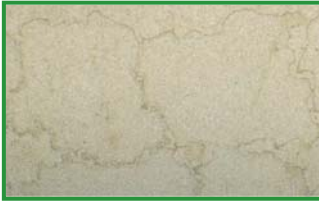
Marbling caused by impurities in steam condensate
