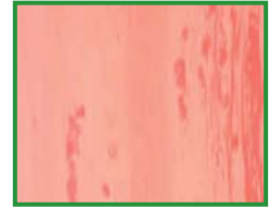
Aluminium surface damage due to use of highly alkaline cleaner
