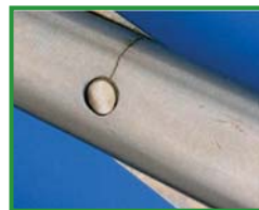
Fracture at hinge
